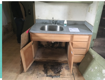
Cervantes Family's kitchen before repairs
